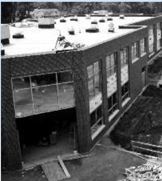
A picture of the CES building project in July. Construction is ahead of schedule and on budget, with students and faculty expected to return in February.
