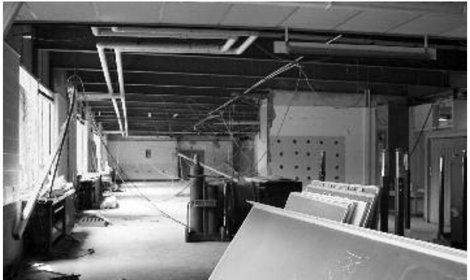
Maple Hill Middle School's library and computer lab were gutted this year so they could be expanded and improved technologically. The rooms will be ready for the opening of the school year.
